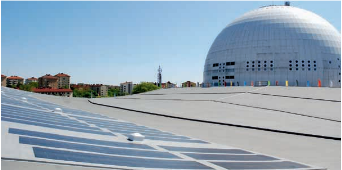
The photovoltaic solar cells on the roof of Hovet sports arena in Stockholm are flexible thin-film modules of amorphous silicon, which are integrated in the roofing membrane. The system supports the illumination for the adjacent Globen arena.
