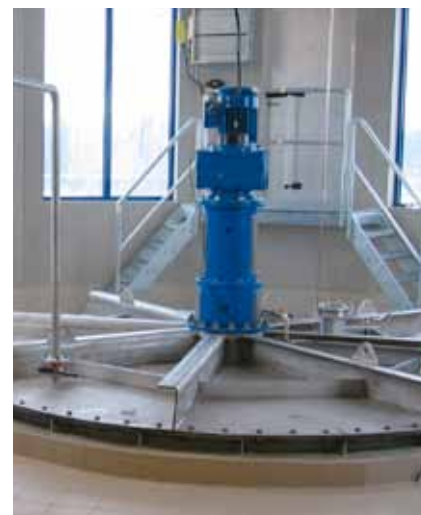
Digester at Purac's waste management plant. Photography from Purac.
